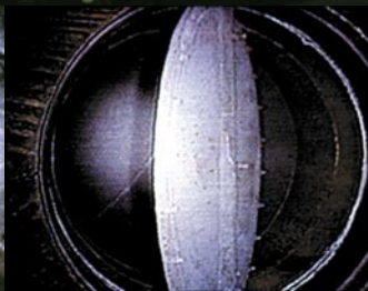
Butterfly Valve – Monitor Operation
